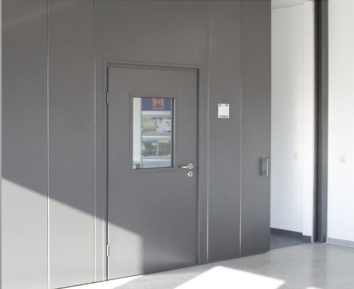
Picture 15: Wicket door with integrated overhead door closer
