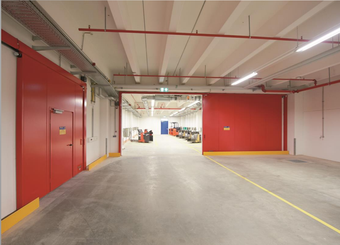
Picture 6: Fire-& smoke- tight sliding door in a warehouse coated in RAL 3000
