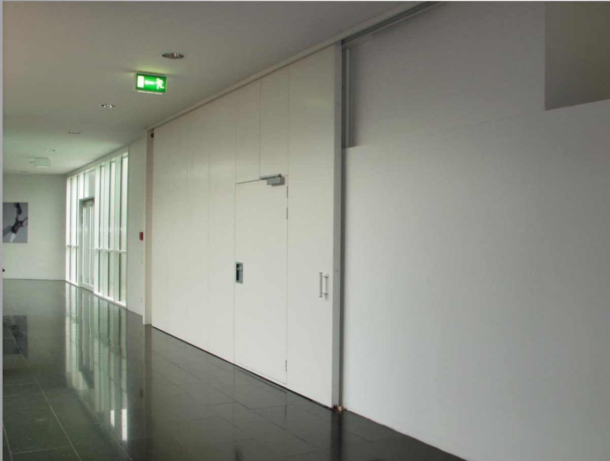
Picture 5: Fire- & smoke- tight sliding door with wicket door in a school building
