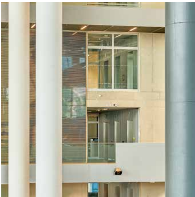
Fixed fire-rated and smoke-tight glazing seen from the atrium.
