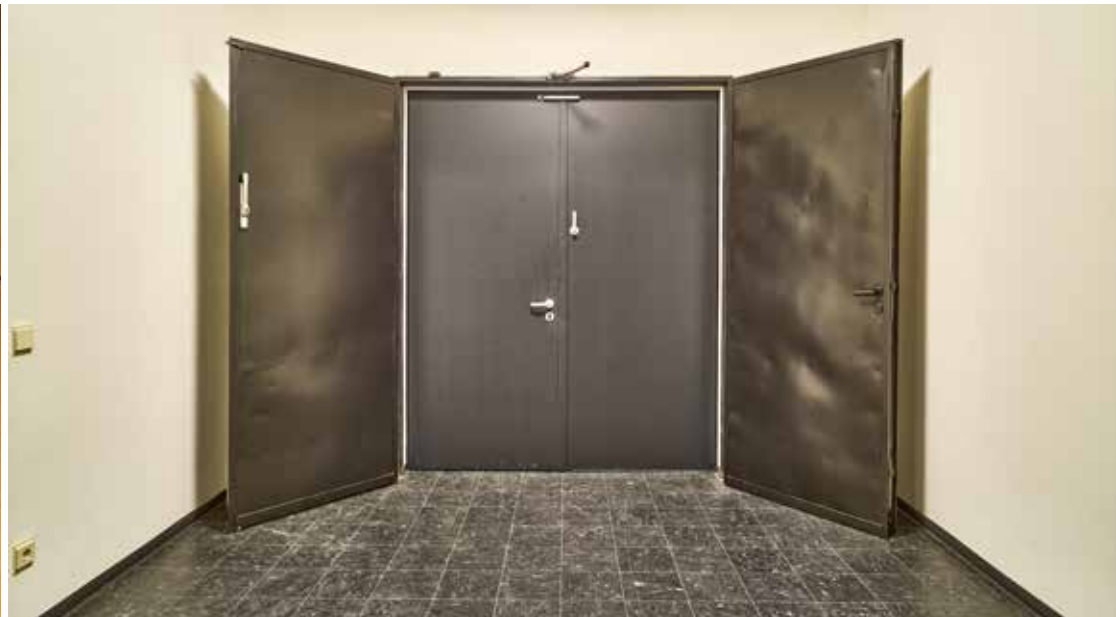
The historic sheet steel door has been preserved and joined by a fire-rated door to form a double door system.
