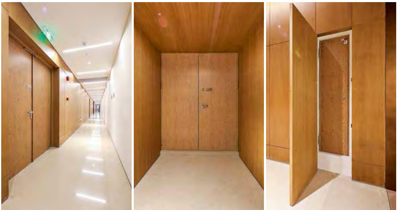
An oak surface finish hides the fact that these doors are actually steel fire-rated doors.
